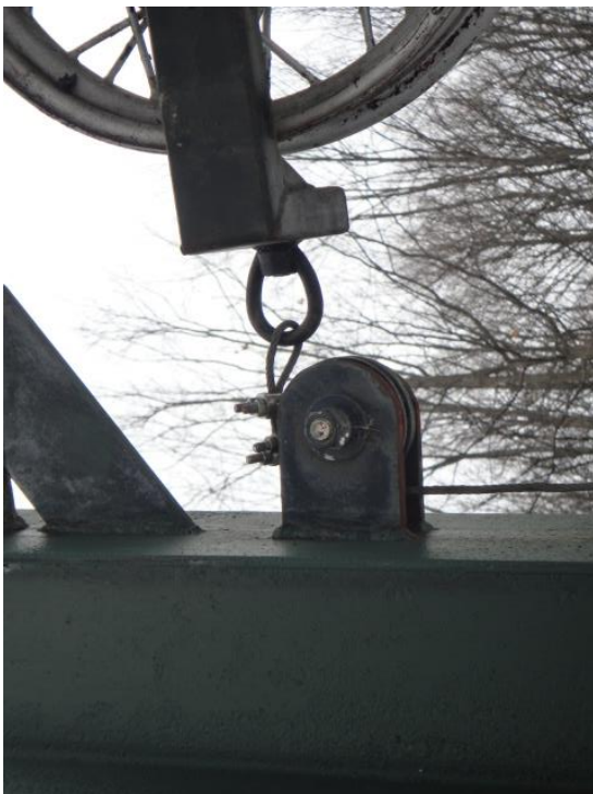
Tension Cable Idler Wheel (Garage Door)
