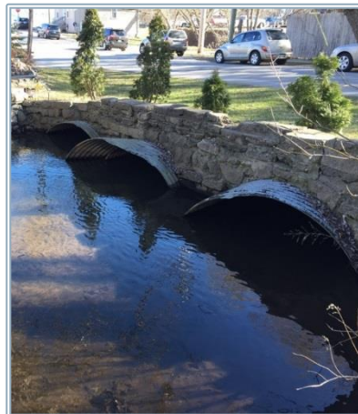
Figure 2. Upstream of the lower Cedar Street Crossing (note sand deposition and culvert filling)
