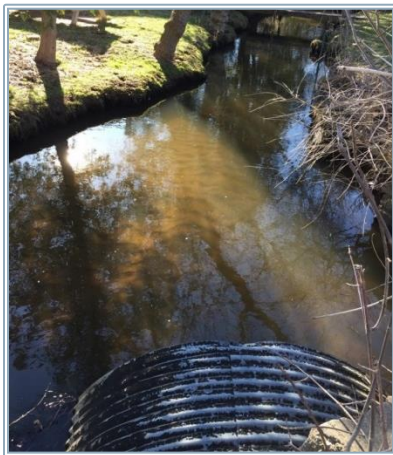
Figure 1. Looking upstream from the Upper Cedar Street crossing (note heavy sand deposition)
