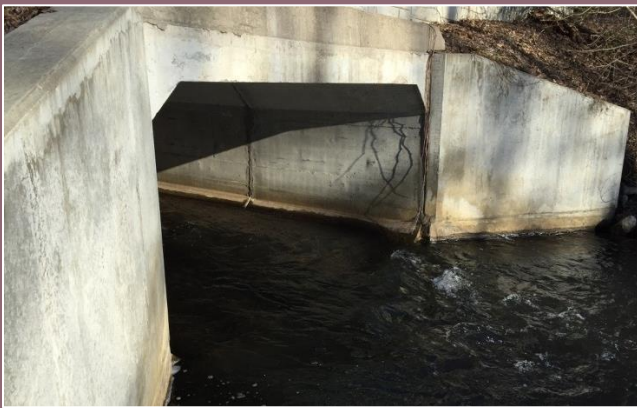
Figure 20. Downstream end of Kids Creek (Wadsworth Street culvert) at the Boardman River. Flow depth is less than 6-inches deep
