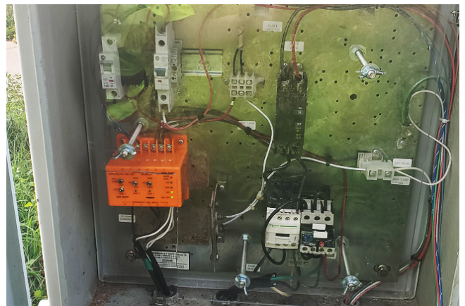
Hull Park control panel reconfiguration.
