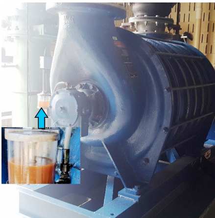
Blower 1 seal fail.
