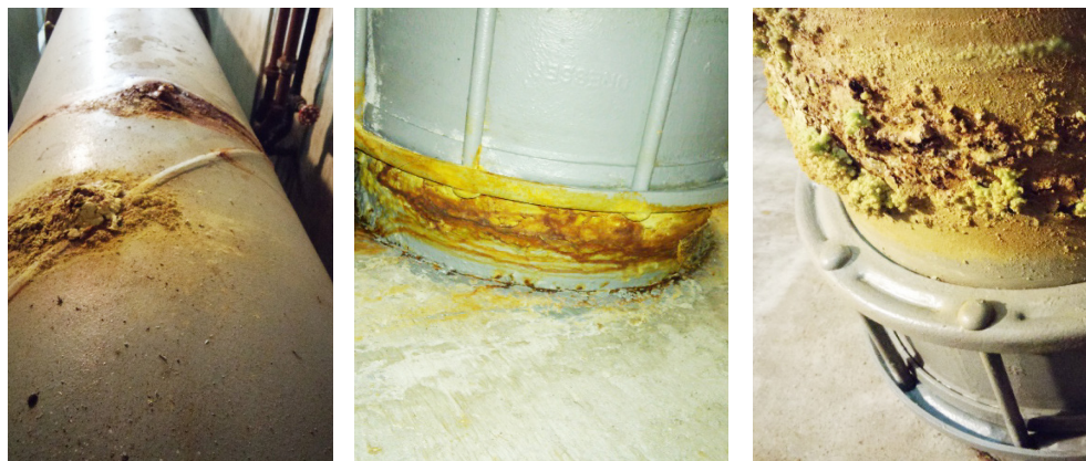
Primary header installed in 1976.
