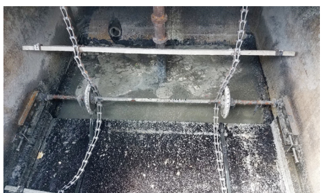
Inside a clarifier tank installed in 1932.
