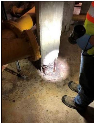
Photo 10- Deteriorated concrete w/ exposed reinforcement at column base
