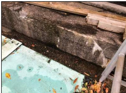
Photo 8- Deterioration along grit chamber walls
