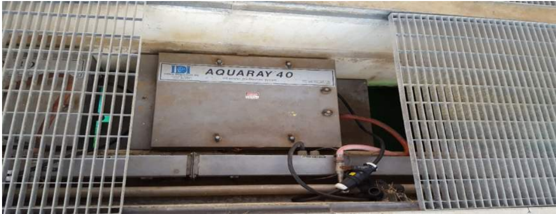
UV Module in Channel
