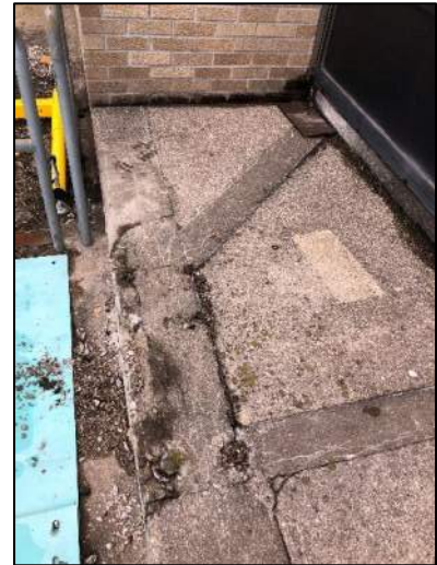
Photo 4- Deteriorated concrete along top slab of grit chamber
