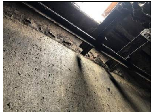
Photo 7- Coating failure at waterline
