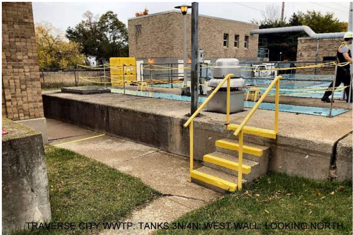
Figure 1. Views of the Traverse City WWTP facility in October 2014. The top view shows the tanks labeled 1S and 2S. Core 1S-1 was taken from the vertical wall separating Chamber 1S from 2S (1930s construction). The bottom view shows Tanks 3N and 4N. Core 3N-1 was taken from Tank 3N, which was constructed in the 1960s.
