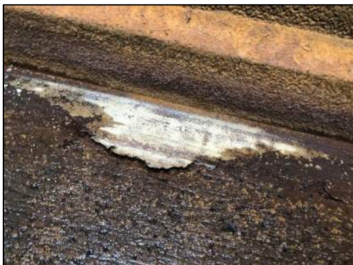
Photo 3- Concrete slab beneath hardened sludge
