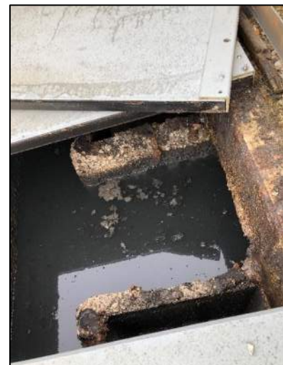
Photo 6- Cement paste loss and exposed aggregate at scum troughs
